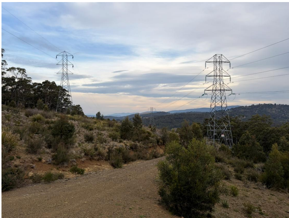
Figure 33: TasNetworks high voltage transmission infrastructure that runs through an easement on a significant portion of the property.
