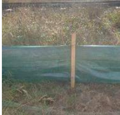
Figure 6: Temporary silt fence 300 mm width with 100 dug into the ground or folded in with rocks placed on the folded side
