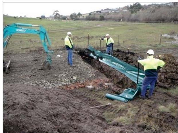
Sump to drain cleandown effluent
