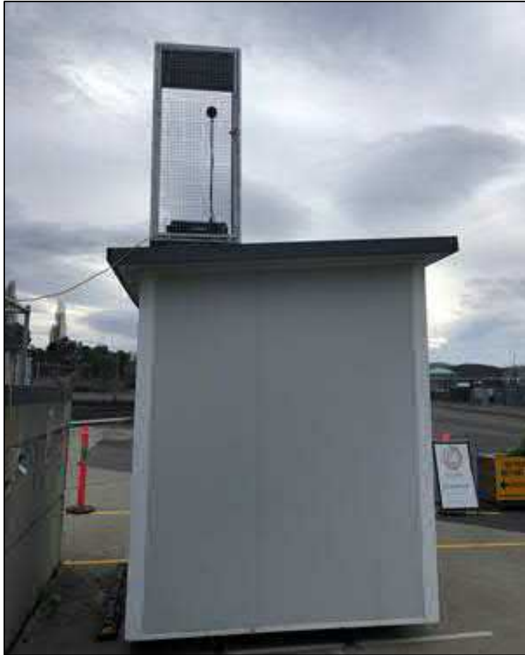
Figure 3. The Corporation's noise monitoring station in the south part of the Precinct near Evans Street.
