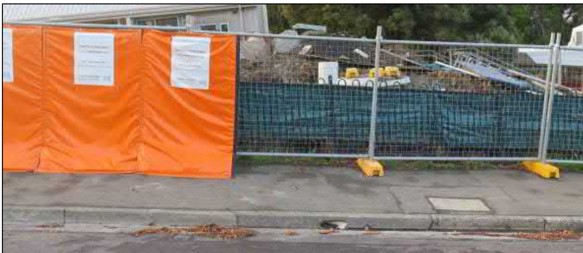
Figure 1 Typical sound absorbing barriers mounted on a temporary fence at a project in Hobart. These barriers are each 2m high and 1.3m wide and they can achieve 12-15 dB noise reduction when placed near a noise source such as a jackhammer. A heavy duty version of the barriers is also available that can achieve much better performance, especially regarding low frequency noise. There are other similar products on the market.
