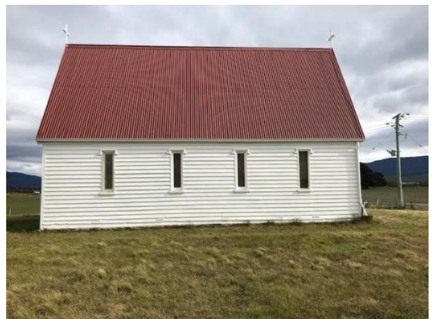
North side of the building with 4 equally spaced narrow windows. The weatherboards extend to the ground with no visible foundation wall
