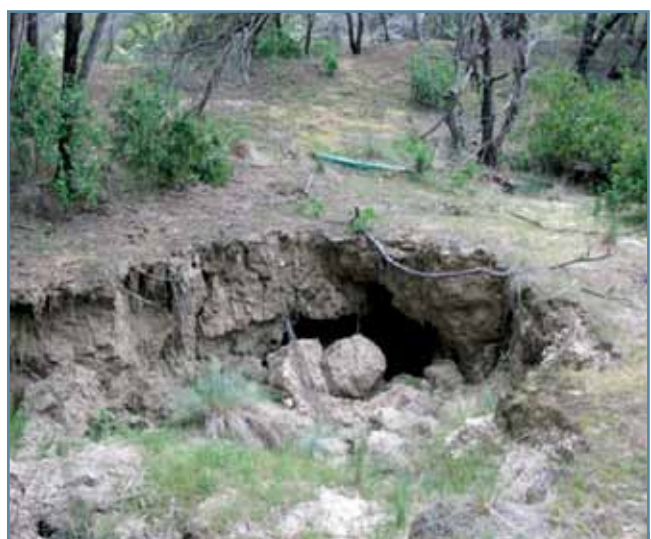
Figure 34. Piping failure of a dam constructed from soils derived from Permian mudstone, Penna area. This dam is known to have failed on first filling. The image was taken from the dam floor, looking at the inside of the dam wall.
