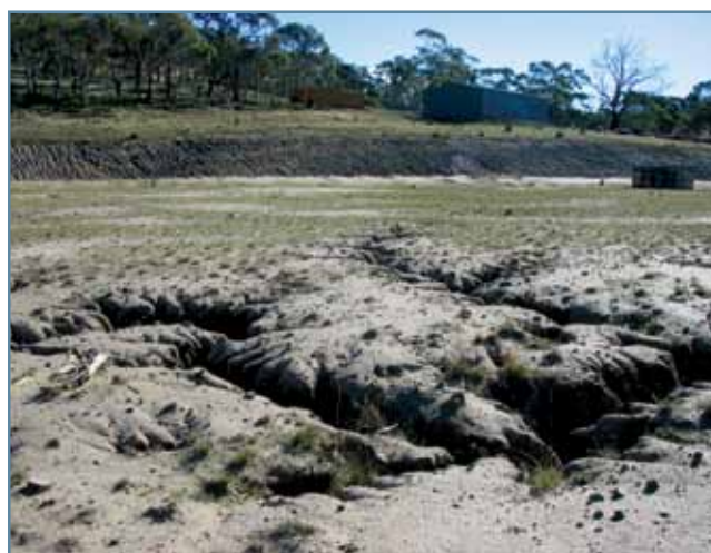
Figure 18. (Same site as Figure 17) Tunnel erosion in footings intended for a large building. Erosion resulted from ponding of rainwater on highly dispersive fill. The fill contains a number of narrow slots (up to 1.2 meters deep) caused by surface water 'dissolving' through the footing.
