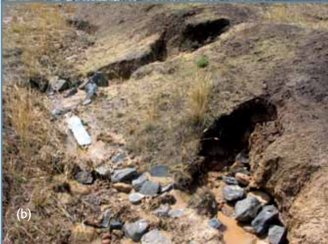
Figure 26. Undercutting and collapse of roadside batter due to construction of a table drain in dispersive clay. Note the failure of the blue rock rap to prevent further erosion.
