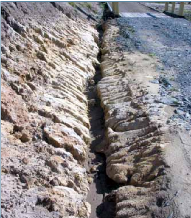
Figure 27. Table drain constructed in dispersive subsoil. The concentration of runoff in the culvert is greatly adding to the erosion problem, resulting in slumping and undercutting of the road and the adjacent batter slope. This photo was taken 18 months after the driveway was constructed.
