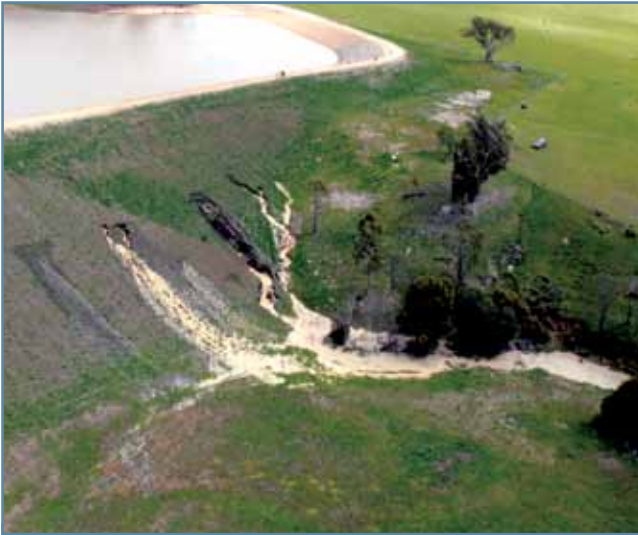
Figure 35. Failure of Blackman Creek dam (source: Davies Brothers). In 2005 the Blackman creek dam failed, resulting in the evacuation of Tunbridge. Doyle and Cumming (unpublished 2005) indicate the cause of the failure to be variability in the compaction of a slightly to a moderately dispersive soil layer, combined with rapid filling of the dam with low electrolyte water.
