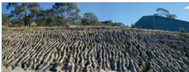
Figure 17. Extensive 'outlet initiated' tunnel and rill erosion caused by excavating a cut and fill pad for a large building in a dispersive soil. Triassic sandstone parent material.
