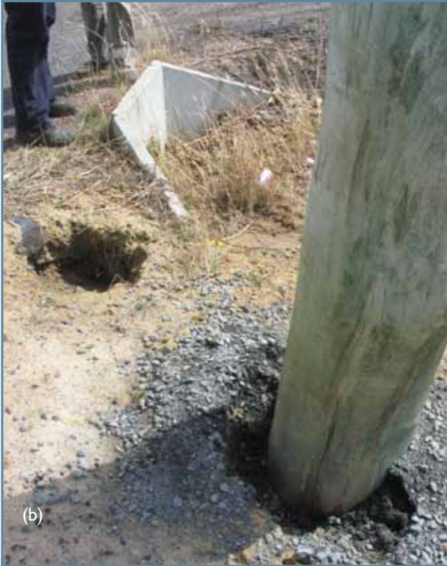
Figure 21 (a) Tunnel erosion initiated by installation of an optical fibre cable into a dispersive soil. (b) Subsidence and early stages of tunnelling resulting from inappropriate installation of power pole in a backfilled trench.
