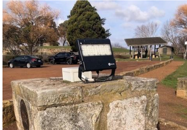
Ross Bridge flood light
