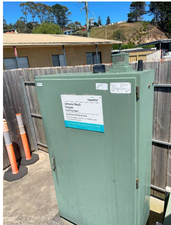
Image 2: Switchboard, Installed January 2013
