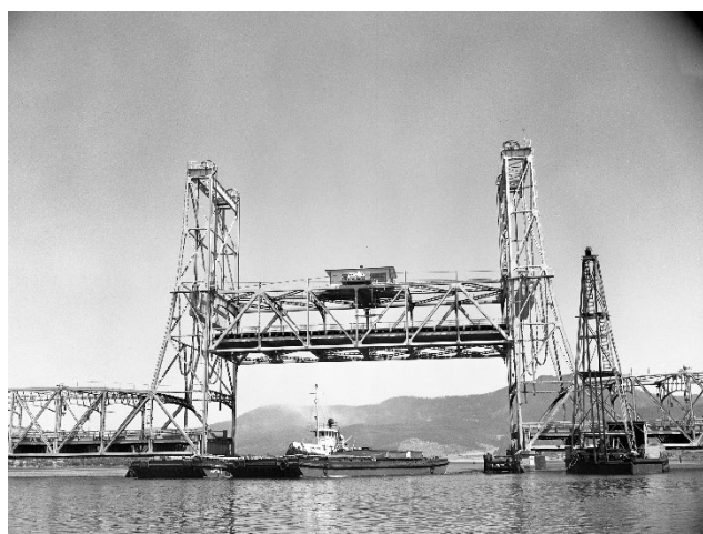
Figure 5 Bridgewater bridge – a vertical lift, Pratt truss through bridge. (Source: 'Tugboat with barges from APPM Boyer passing under the Bridgewater Elevator bridge' , 1957, TAHO, AB71311/5575)
