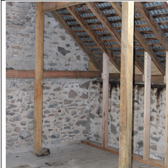
Figure 4: Interior of first floor showing timber roof and flooring construction with stone walls
