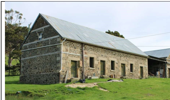
Figure 2: View of front East façade of Rheban Stables – with annex on the right
