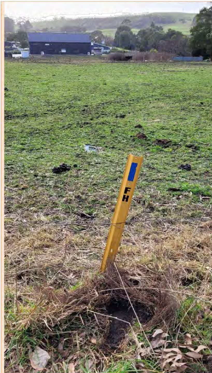
Existing fire plug adjacent to Lot 11 on Golf Links Road
